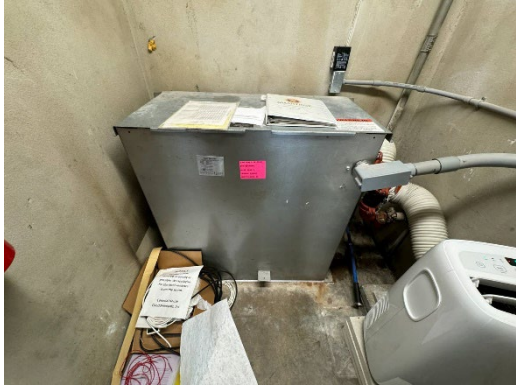
View of Elevator Equipment
