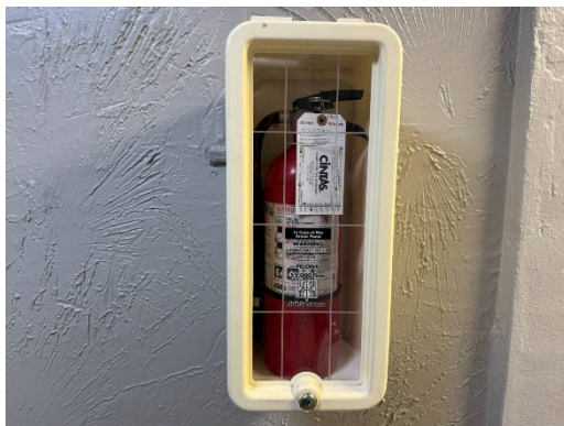
General View of Fire Extinguisher
