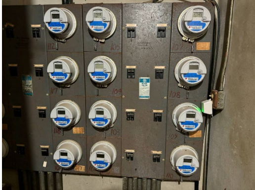
View of Electrical Equipment
