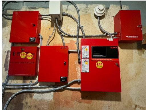
View of Fire Alarm Control Panel
