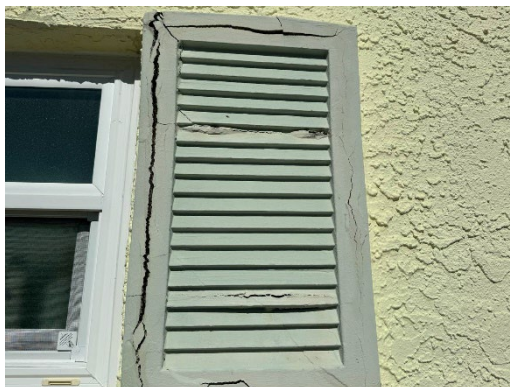
View of Deterioration to Cosmetic Shutters
