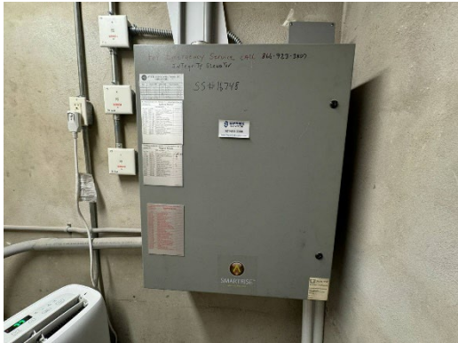
View of Elevator Equipment
