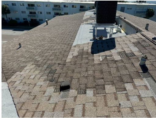
View of Missing Shingles
