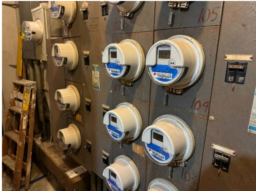
View of Electrical Equipment
