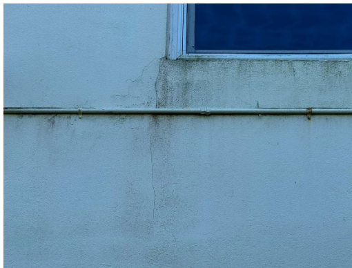
View of Minor Stucco Cracking
