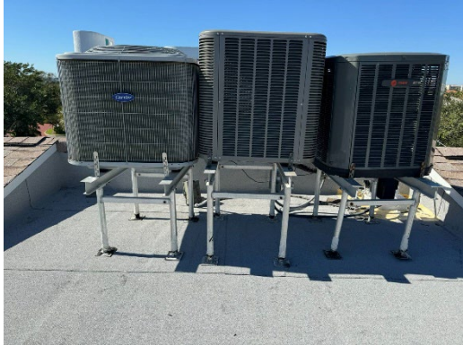
General View of HVAC Equipment on Rooftop
