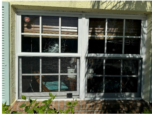
View of Damaged Window
